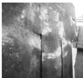
图6 钢板破坏图 Fig.6 Failure of steel plate
