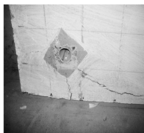
图7 混凝土板角部破坏 Fig.7 Failure of concrete panel
